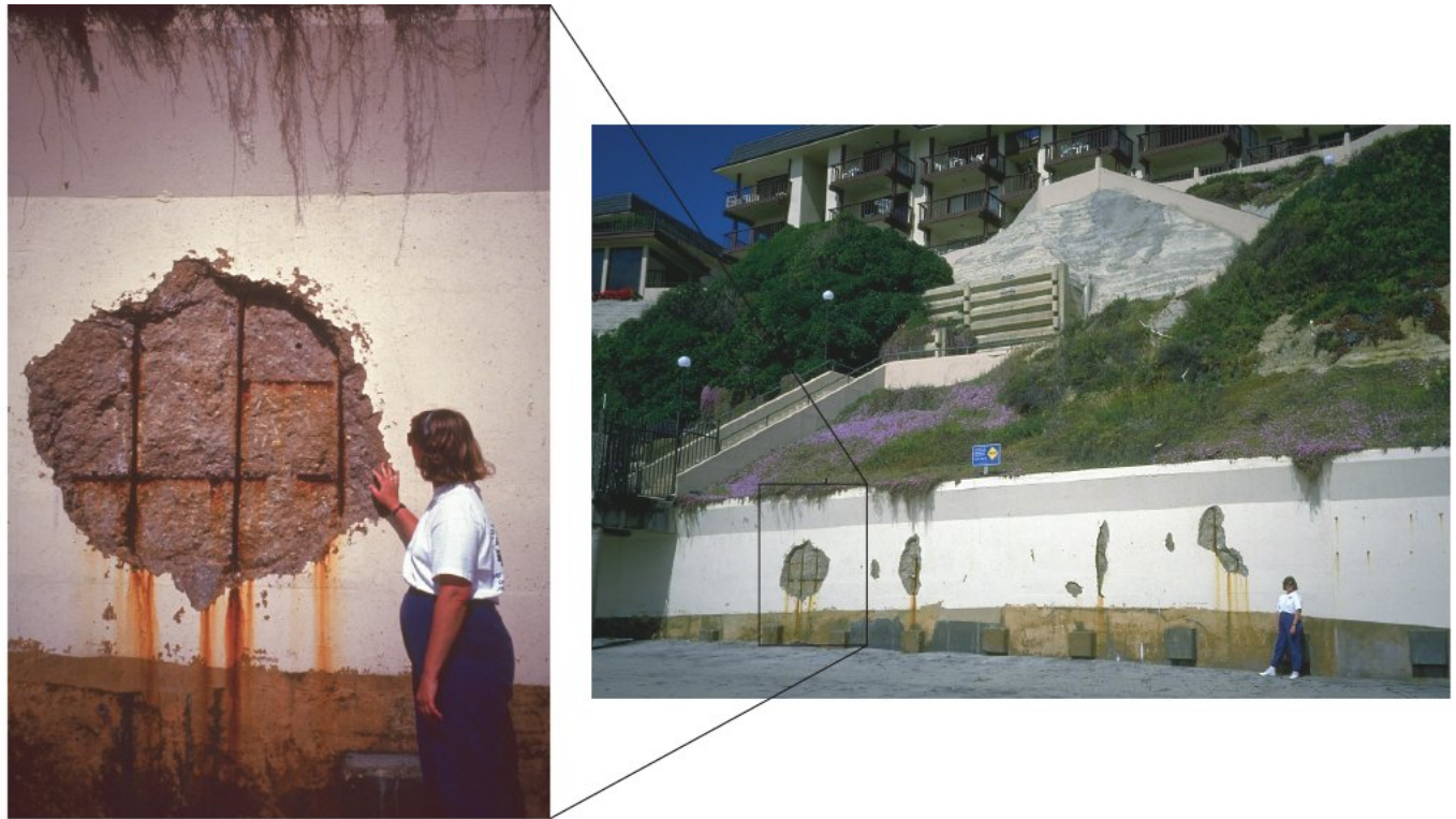
FIGURE 10.25 Seawall damage. A seawall in Solana Beach, California, that has been damaged by waves and needs repair. Although seawalls appear to be sturdy, they can be destroyed by the continual pounding of high-energy storm waves.
